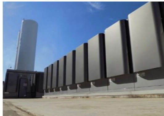
Solid oxide fuel cells at the Fukui site
